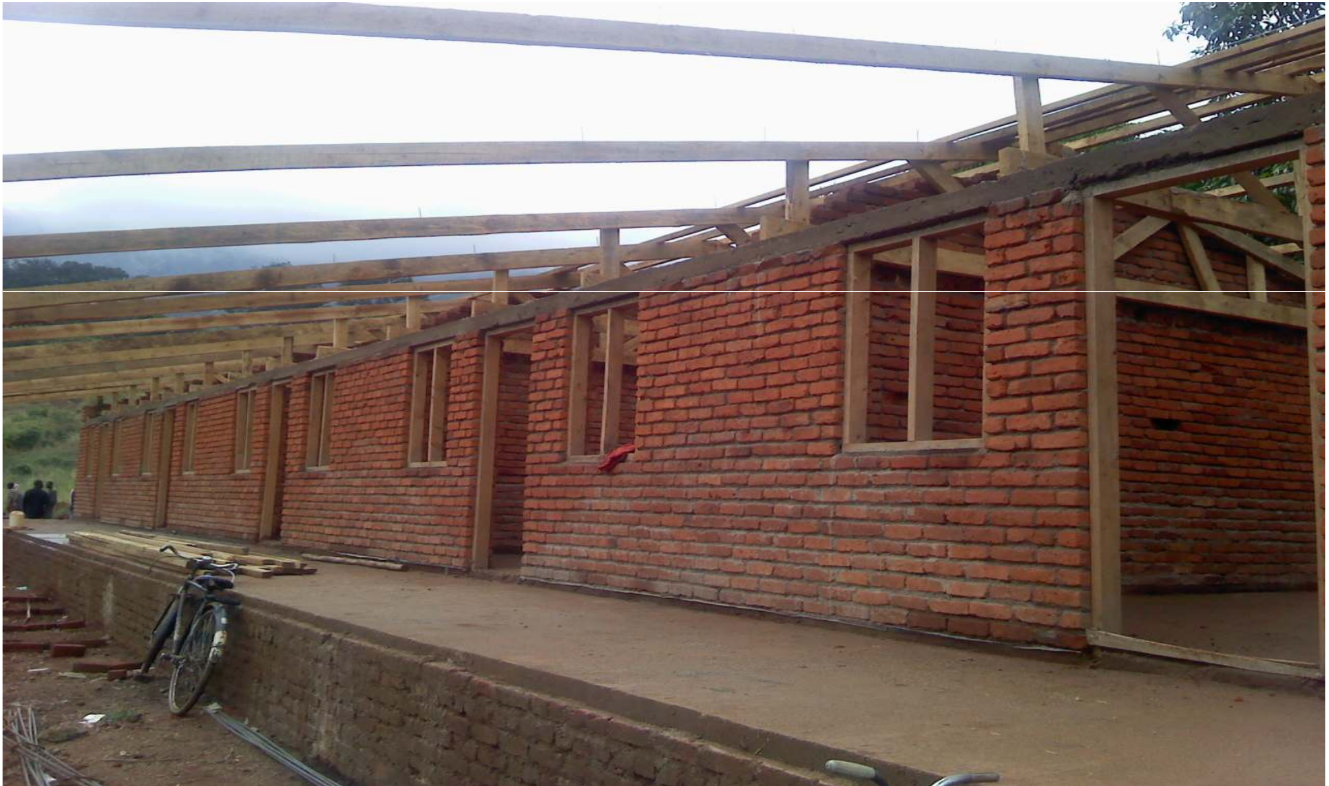
Pic.3: Mens shelter; Front view, about to complete roofing with iron sheets
